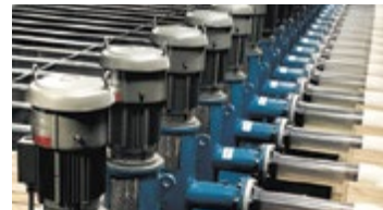
Vertical Pump in Operation
